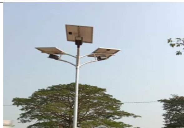
Plate 7.2.4.a. Solar street light
