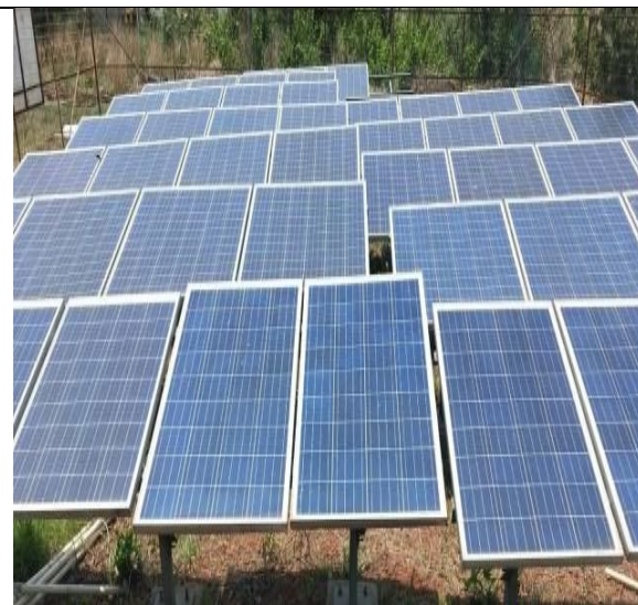
Plate 7.2.4.b 8kW Solar panel
