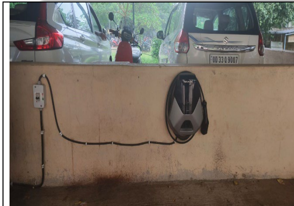
Plate 7.2.4.c. Common charging point
