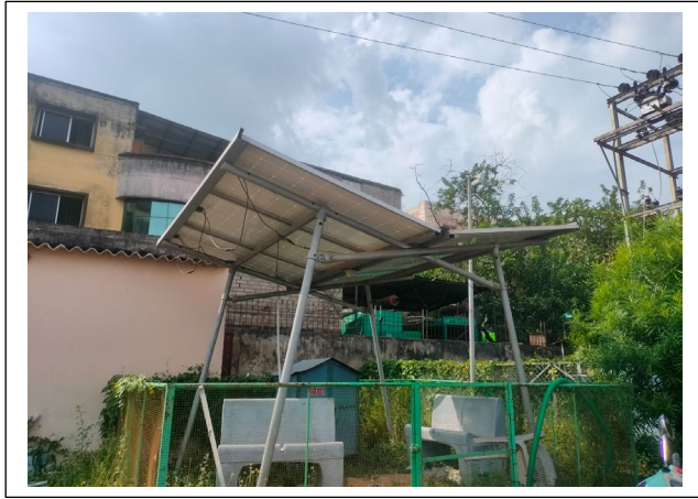
Plate 7.2.3.d 2kW Solar panels for street light
