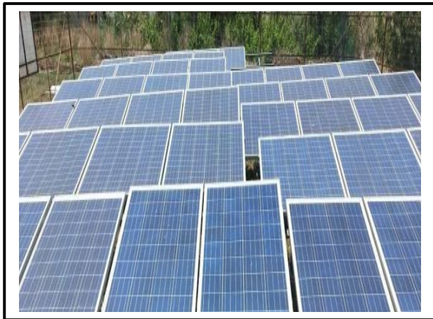
Plate 7.2.2.e. Solar panel system
