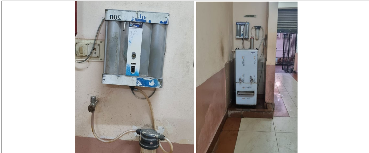
Plate 1- UV water Purifier installed in every floor of the academic building.
