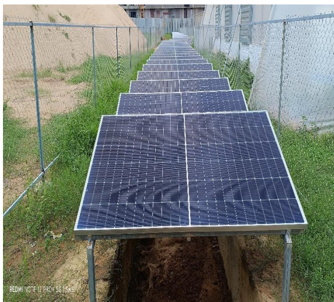
Plate 3- Solar panel on rainwater trench system
