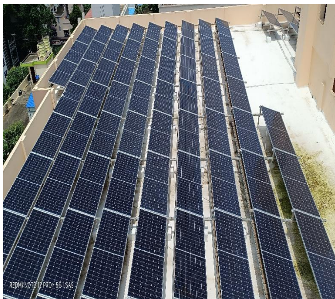
Plate 1- Solar panel of 580kWp
