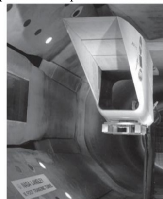
Fig 15:- The SAMPSON inlet cowl as installed in the NASA Langley Transonic Wind Tunnel
