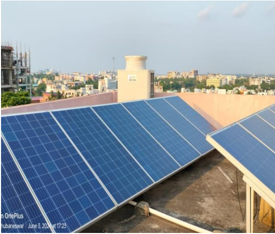
10 kWp Solar Plant
