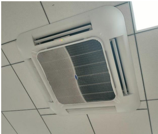
Cassette ACs for power saving
