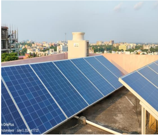
10 kWp Solar Plant
